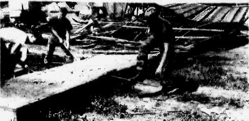
PFC Randy VanMarteir (l), Cpl. John Corpus, and LCpl. Timothy Aherns, reservists from WES-40, break up the floor boards of a demolished supply shed taken down in the 3d Marines' area.
