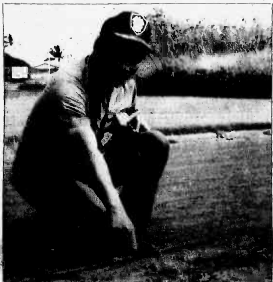
Robert Meheula, of the Athletic Maintenance Crew, points to the ruts left on the Pop Warner Field track by mopeds and bicycles.
