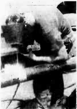
LCpl. Richard Koenig, a reservist with WES-40, welds poles together for the golf course safety screens.
