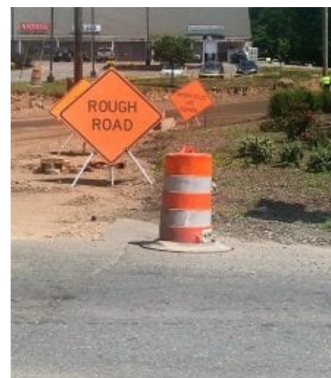
Construction work on Southwick's Congamond Road is slated to continue through November. (Photo by Hope E. Tremblay)
