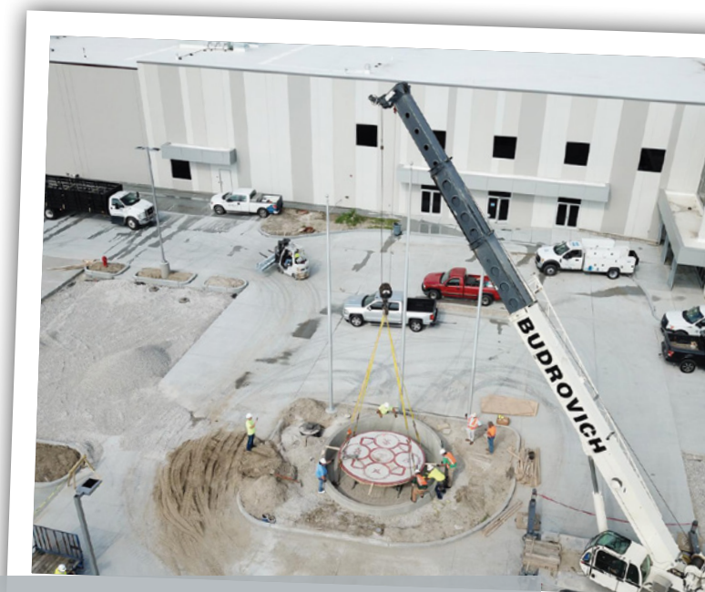
The 50-year-old, 8-ton ornamental Local 562 logo that had been etched in the bottom of the pool at the local's former recreation complex in Spanish Lake is installed in its new home at the local's future training center on June 3, 2020, as the centerpiece of a monument in front of the facility at 3755 Corporate Trail that is set to open in the summer of 2020. The pool had been filled in about 15 years earlier, but the logo was extracted and placed near the first tee at the union's Emerald Green golf course and was later placed in storage.
