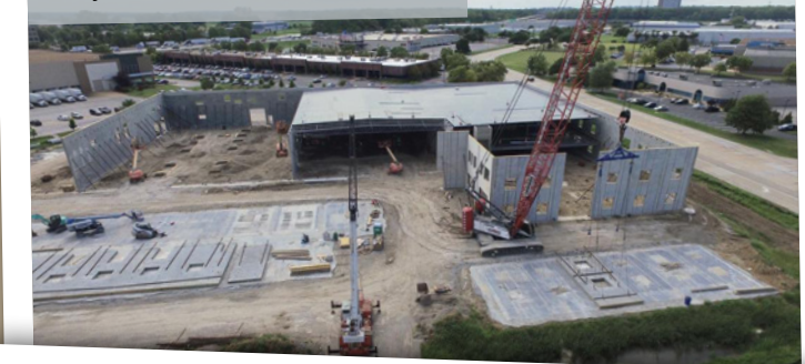
The new Local 562 training center in Earth City under construction in August 2019.
