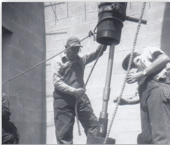
Local 562 members work on construction of the new Meramec Power Plant in south St. Louis sometime during the late 1950s.
