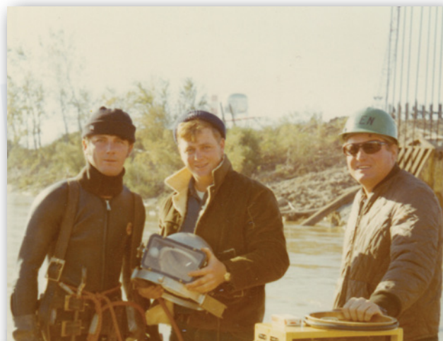
Local 562 Brother John Lane is assisted into his diving suit for a dive to work on an underwater inlet structure during construction of the New Madrid Power Plant in New Madrid, Missouri, in 1970.
