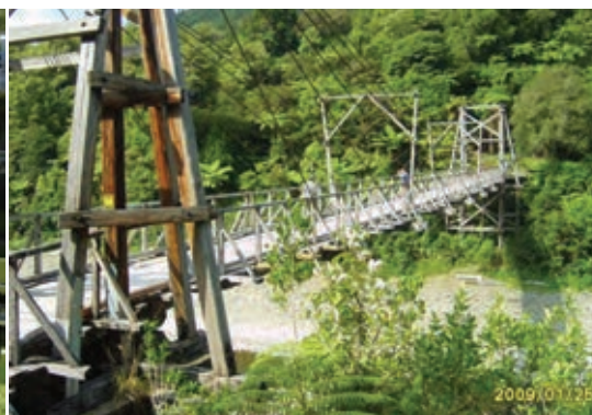
Tauranga Bridge: One of only two remaining single span suspension bridges, located in the Waioeka Gorge.
