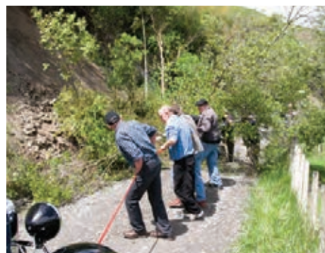
Manawatu: Removing a tree to make a gap through the slip on the Burma Hill Rd.
