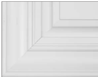
Example of front joint separation
