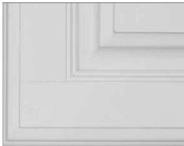
Example of front joint separation
