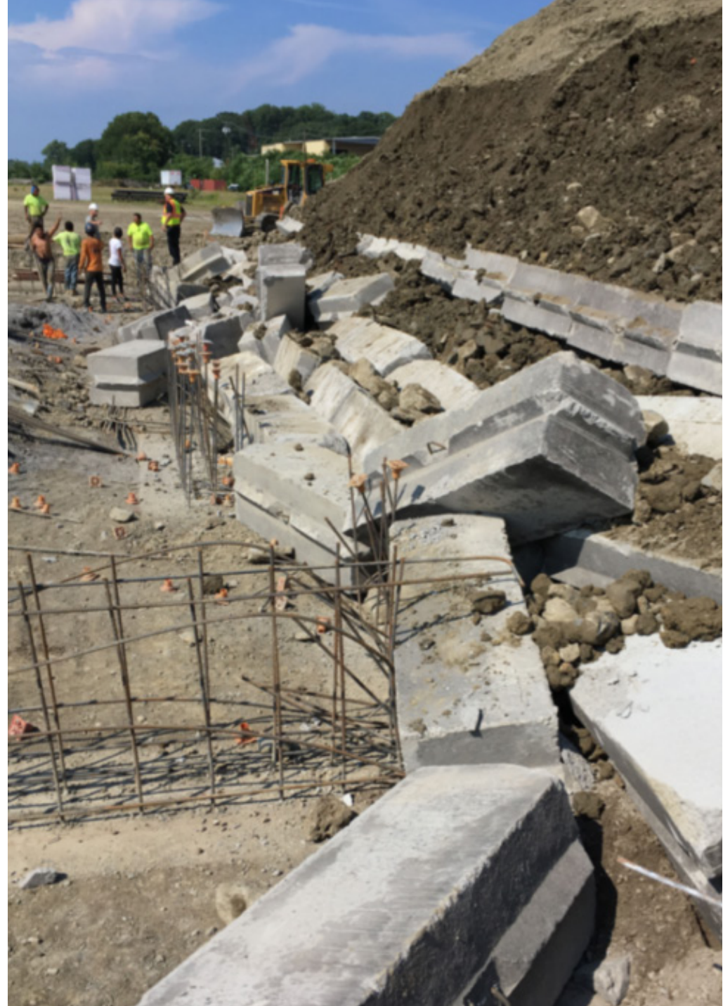
Collapsed wall at Poughkeepsie job site, 2017.
