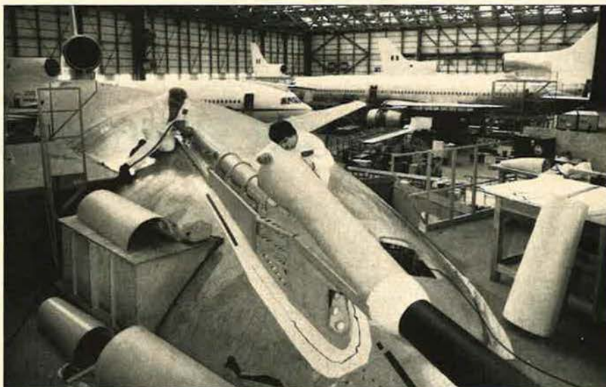
Technicians install a unicorn-like refueling probe to the top of one of the commercial Lockheed L-1011 TriStars that Marshall of Cambridge (Engineering) Ltd. is converting into tanker/freighter aircraft for the Royal Air Force.
