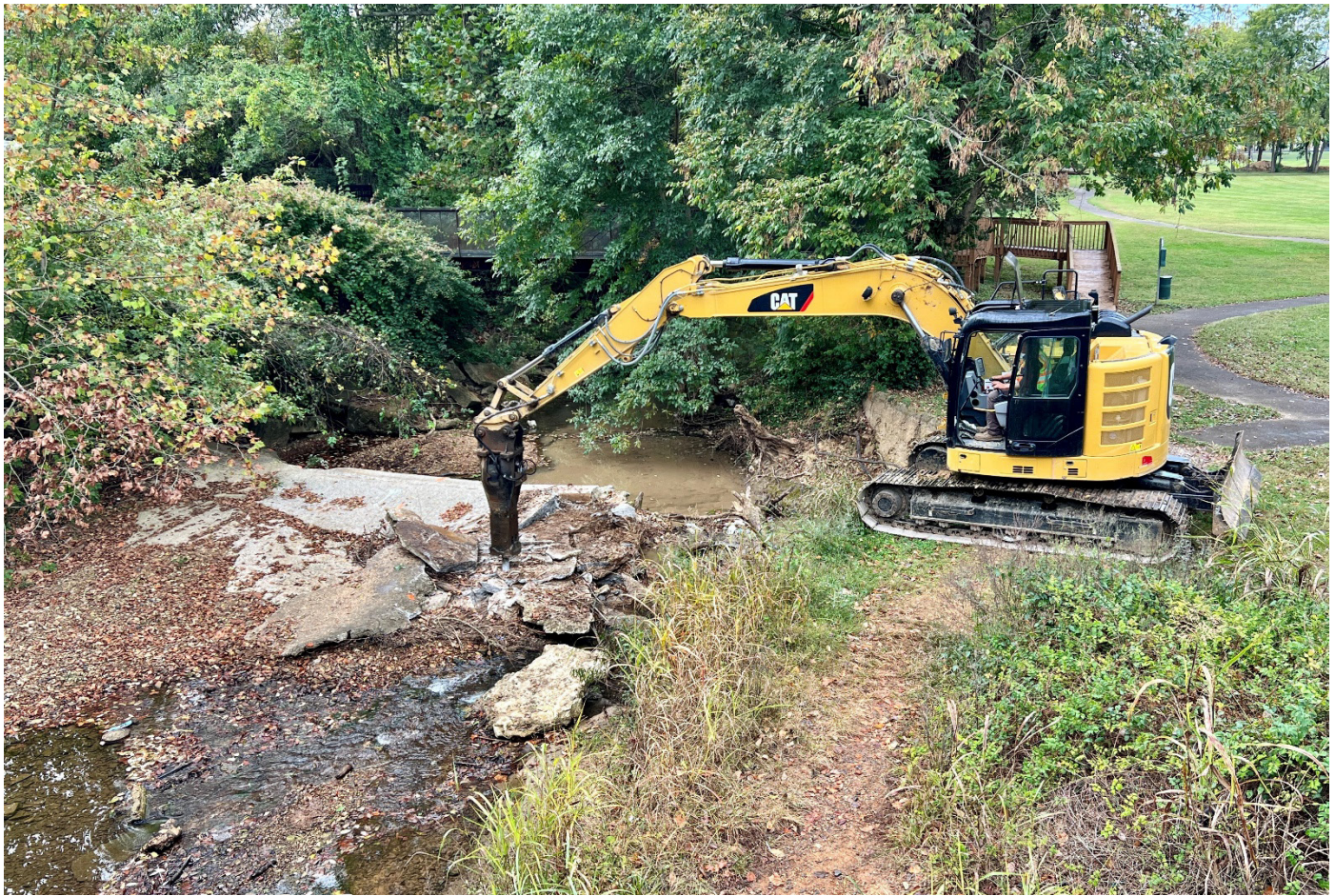
City of Vine Grove Weir Dam, Brushy Fork, KY; Photo Credit: Ward Wilson
