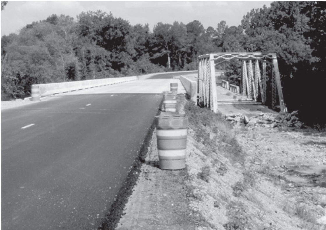
Approximately 560 bridges were to be improved or replaced under the Highway Improvement Program.
