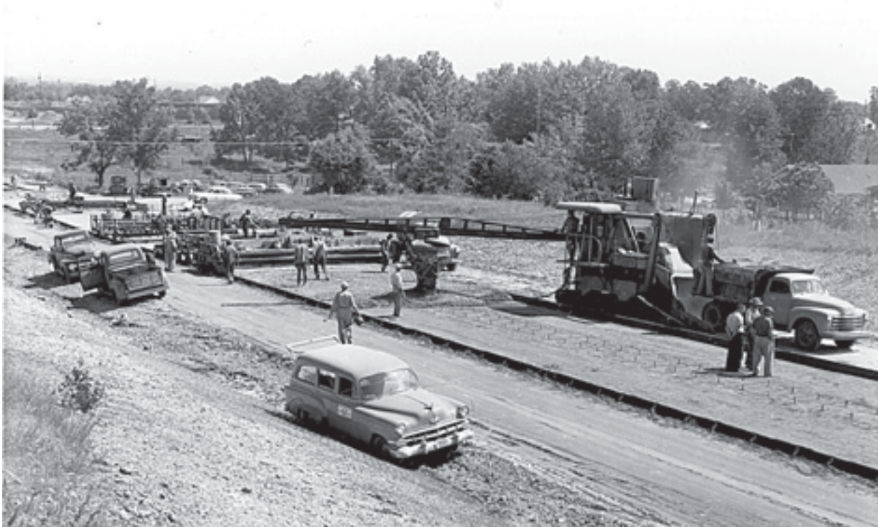
Construction in 1954 on the southbound lanes of the New Benton Highway which became Interstate 30.
