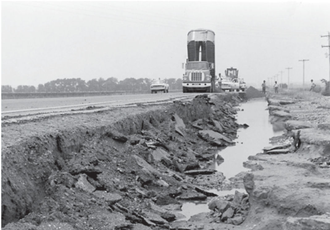
State Highway 41 shoulder damage after the 1990 flood.
