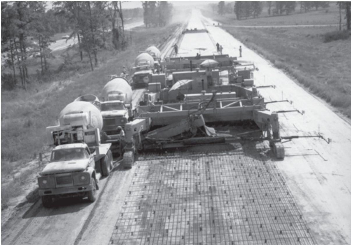
Slip form paving on Interstate 30 near Hope as seen from the Highway 4 overpass in 1970.
