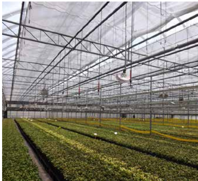
Gutter to Gutter System
