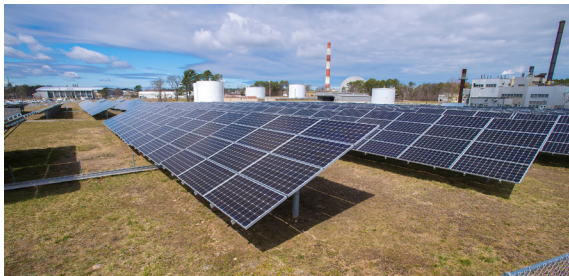
View of the Northeast Solar Energy Research Center (NSERC)
