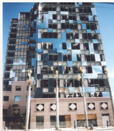
2005 Hurricane Wilma damages Broward County School Board Building Source: Photo by Susan Gillis, Historian
