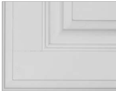
Example of front joint separation
