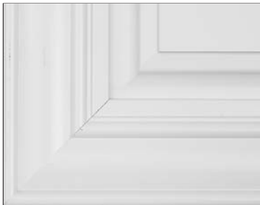
Example of front joint separation
