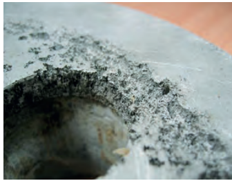
FIGURE 15 Valve body corrosion due to moisture combining with corrosive elements in the gas.
