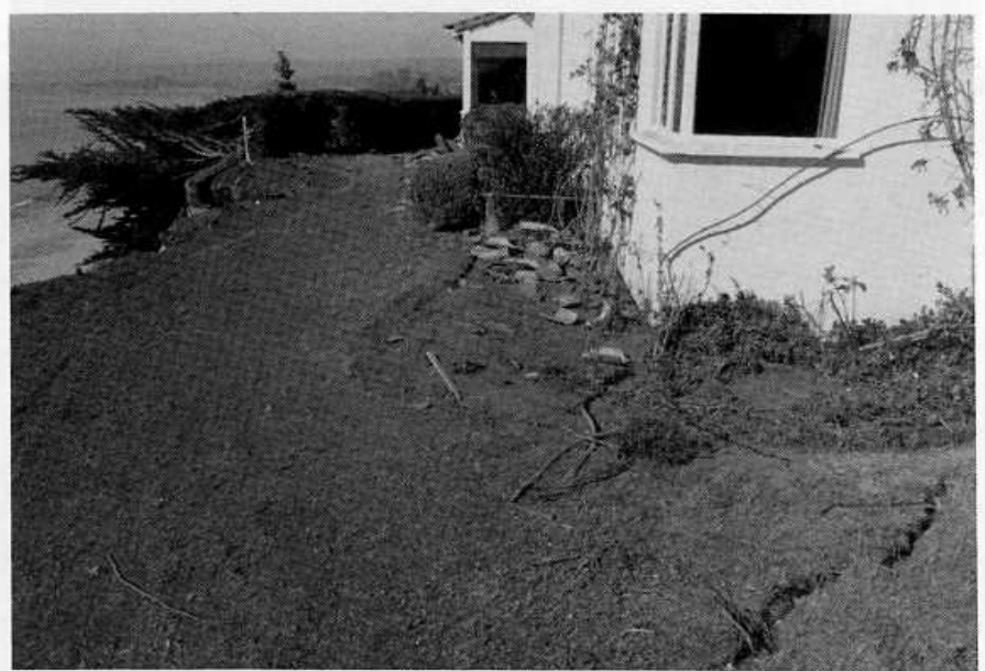
Photo 5. Deep tension crack in terrace deposits. These cracks often cut through house foundations and indicate the potential extent of future failure.
