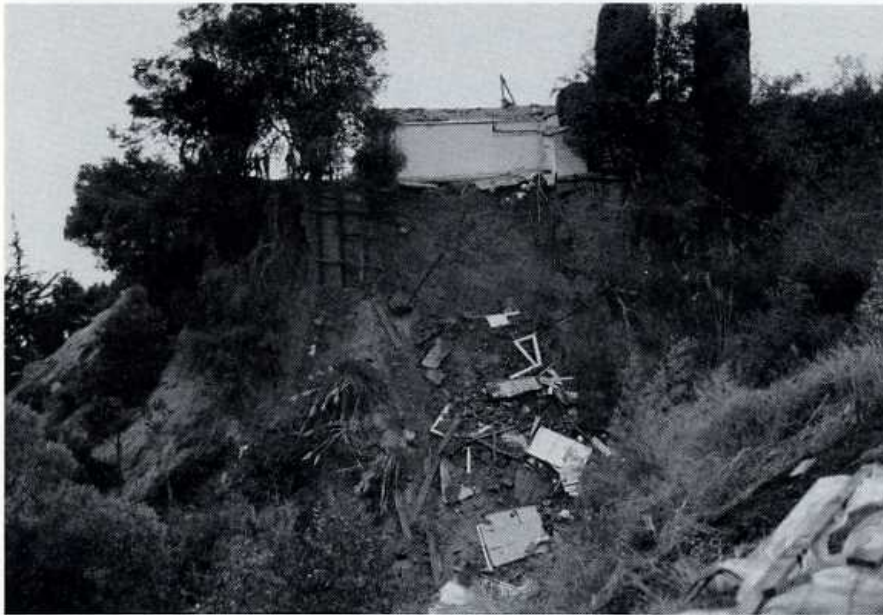
Photo 10. Extensive slope failure and cracking on a narrow ridge. This house will be torn down and the slope will be graded to a safer angle. Houses below this failure were evacuated.
