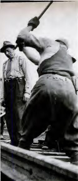
These men are working at the 8-mile point. Under good conditions they have been laying track at the rate of 3,000 feet a day, hope to hit a mile a day by next year.
