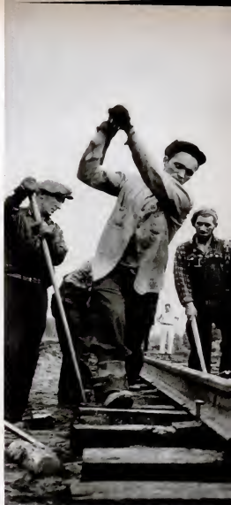
LAYING THE RAILS , members of one of the track gangs, which are usually made up of "Newfies" from Newfoundland, swing their heavy hammers at a spike.
