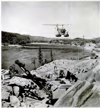
SUPPLIES BY HELICOPTER arrive at camp at Mile 17 which has depended solely on these aircraft during winter. In summertime seaplanes can land on the river and now equipment can be hauled in on a makeshift road from the south.
