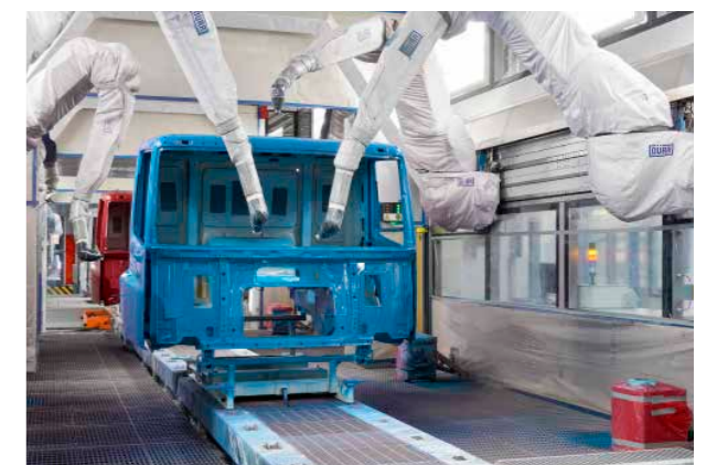
Robots paint cabs in the new state-of-the-art Cab Paint Facility at the DAF premises in Westerlo, Belgium.
