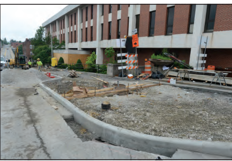
Curbs have been built and bases for the light poles have been set.
