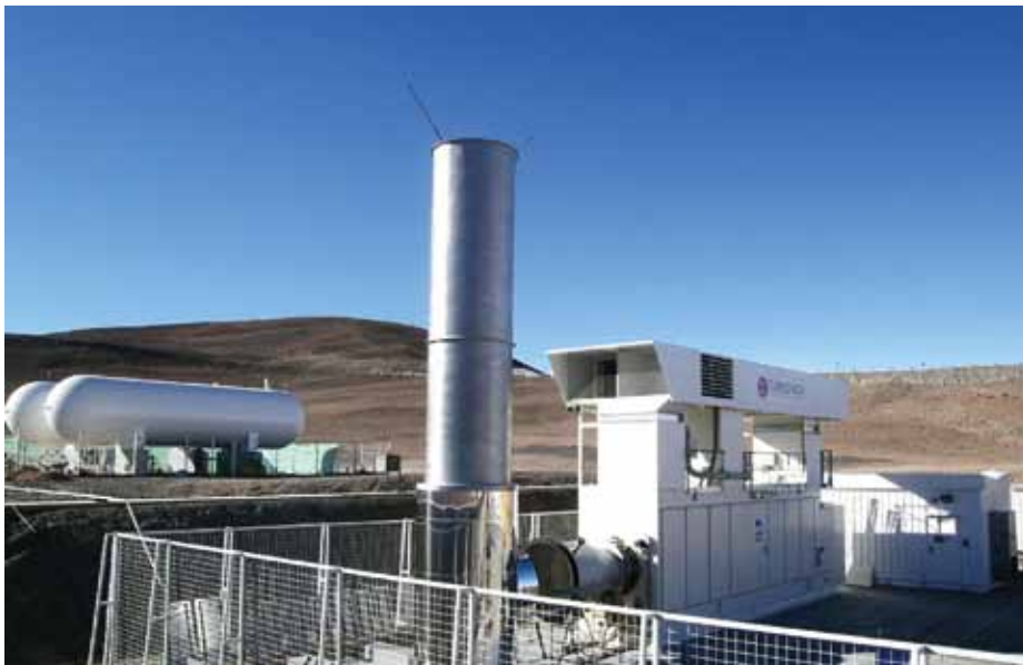
Paranal's new multi-fuel power generator can provide up to 2.2 MW of electrical power. The two tanks for LPG can be seen in the background.
