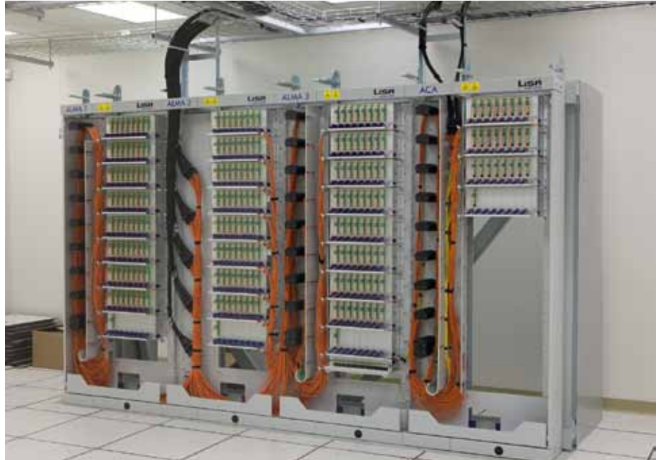
The ALMA patch panel, installed at the AOS. The eight fibres coming from each of the 192 antenna stations are terminated here.
