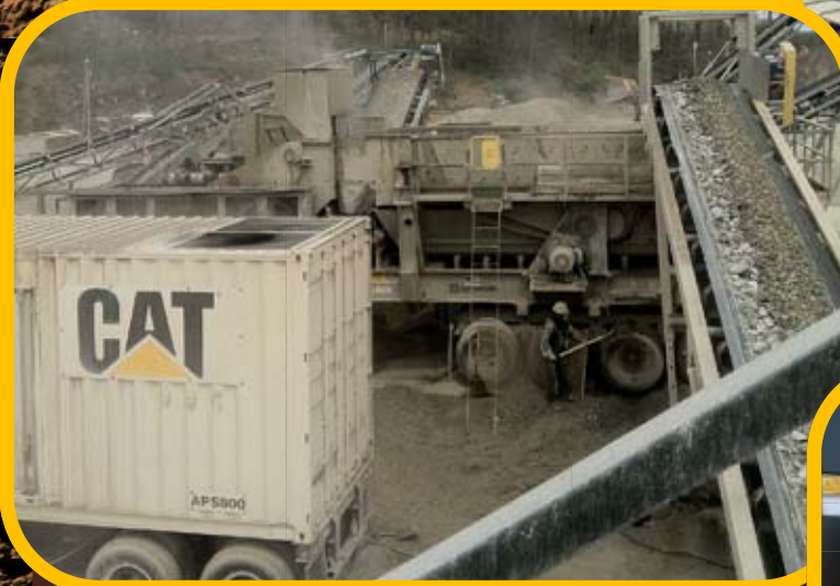
Wantage Stone LLC relies on their fleet of Caterpillar equipment to keep their Hamburg, NJ quarry running at peak performance.
