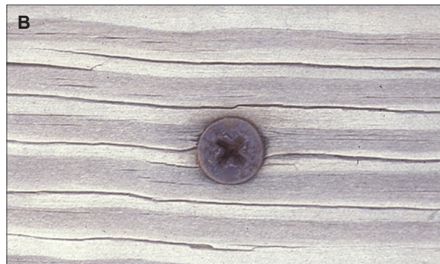
Figure 16–27. (A) Iron stain on newly installed cedar siding. Poor quality galvanized nails corrode easily and, like uncoated steel nails, usually cause unsightly staining of the wood. (B) Pine, on the other hand, does not contain appreciable tannins, so iron stain is not an issue even with rusty fasteners.
