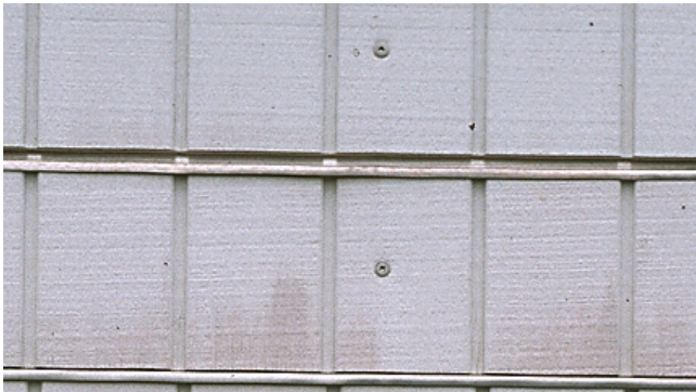
Figure 16-14. Demonstration of proper and improper z-flashing installation: (top) siding installed with a proper 9-mm (3/8-in.) gap between the z-flashing and siding to allow water to drain off the siding; (bottom) siding installed improperly, without a gap. This gives water easy entry into the siding and thus shows extractives staining and promotes decay.
