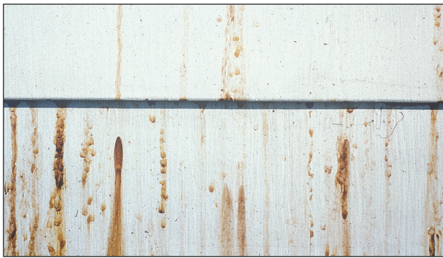
Figure 16–20. Water-soluble extractive discoloration can result from water wetting the back of the siding and then running down the front of the board below.
