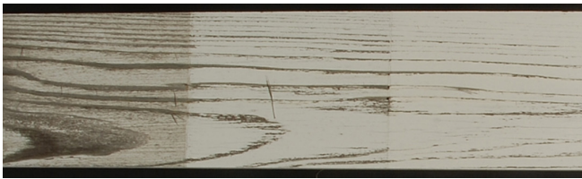
Figure 16-29. Typical peeling and flaking over latewood.
