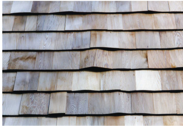
Figure 16–18. Wood shingles installed with insufficient gap, which later buckled when they expanded after getting wet.
