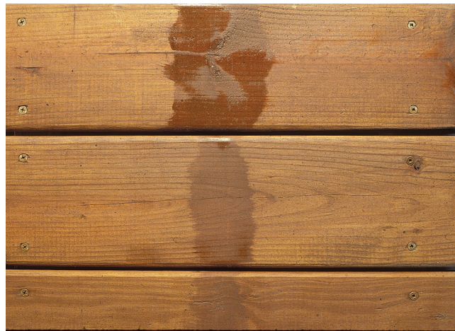
Figure 16–19. Lap marks on wood improperly finished with semitransparent stain.
