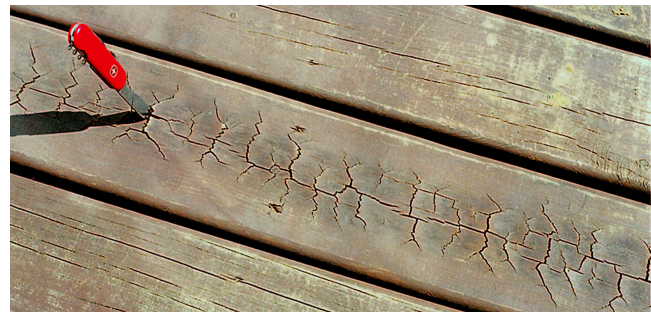
Figure 16–22. Cross-grain checking in juvenile wood. There is no fix other than replacing the board.
