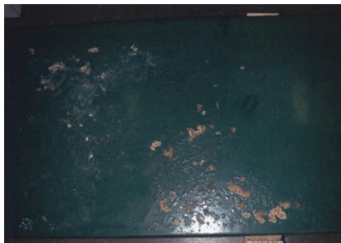
FIGURE 7B Detail of figure 7A showing corrosion.
