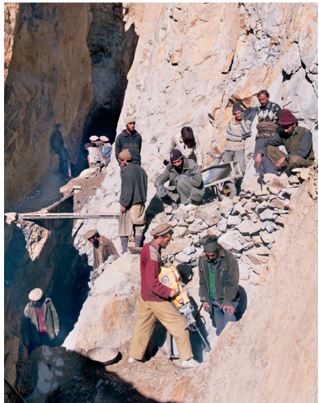
Figure 19. At the Besar deposits, in the Batakundi area of Pakistan's Kaghan Valley, several miners use jackhammers and explosives to break the hard rock in search of sapphires. Photo by V. Pardieu.
