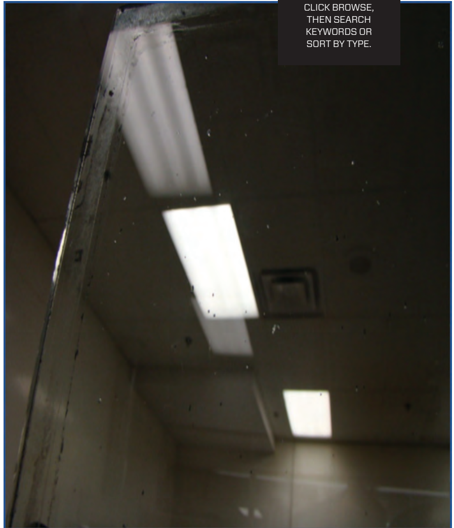
Figure 1. Weld splatter on glass
