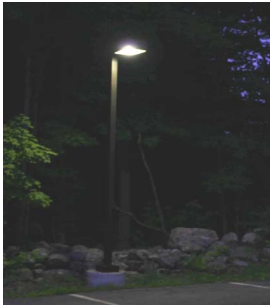
Library parking area – fully shielded lighting directs illumination entirely downward
