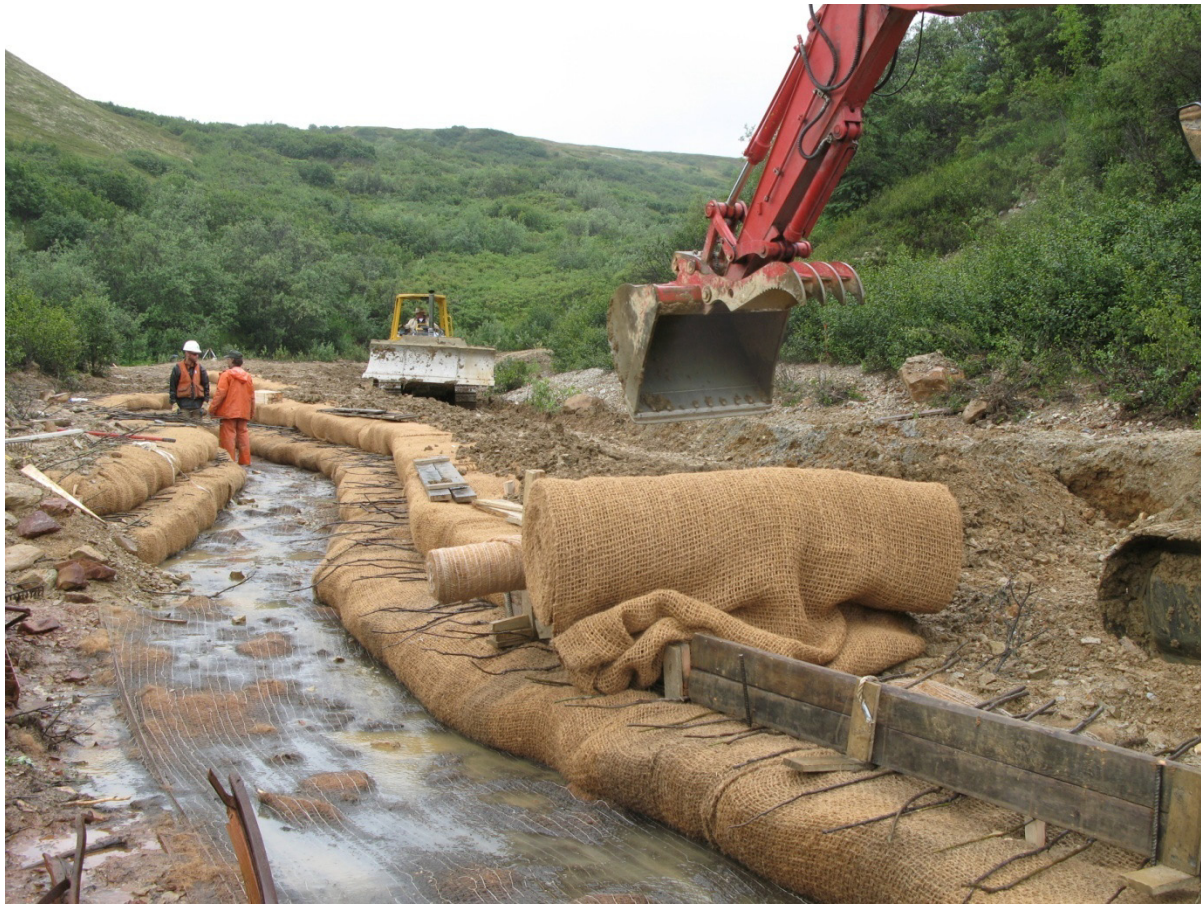
Figure 7: Denali has been steadily restoring abandoned mine lands like this project on Slate Creek. Encapsulated soil lifts guide a new channel away from exposed ore to improve water quality and aquatic habitat. NPS Photo/Adema.
