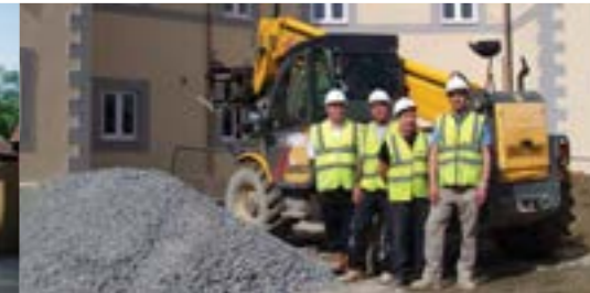
Hills own site foremen work with trusted contractors to deliver sites on time and on budget.
