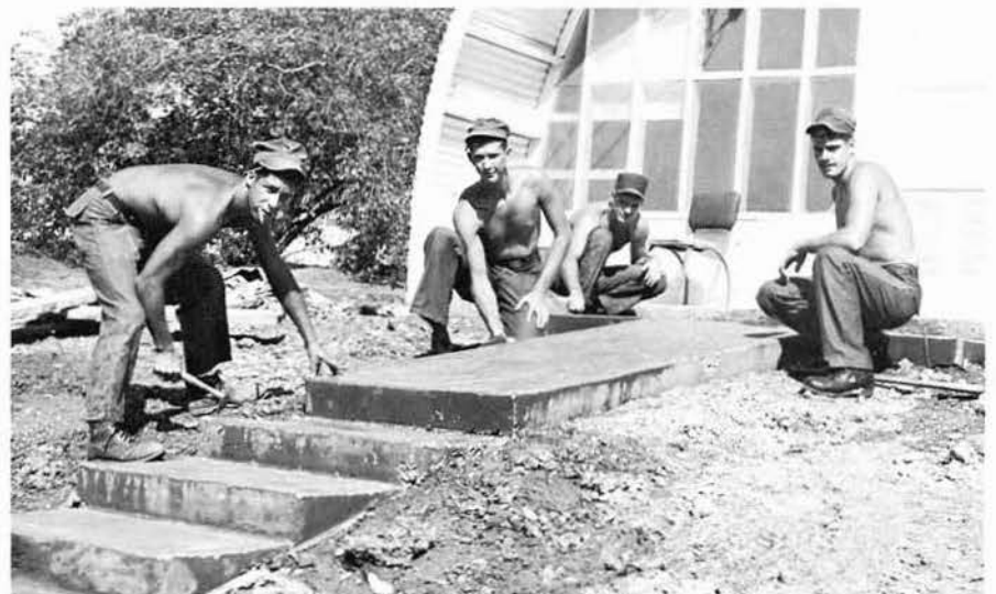
And it came to pass, concrete was delivered unto us, and Bravo disciples went forth to spread the tidings.
