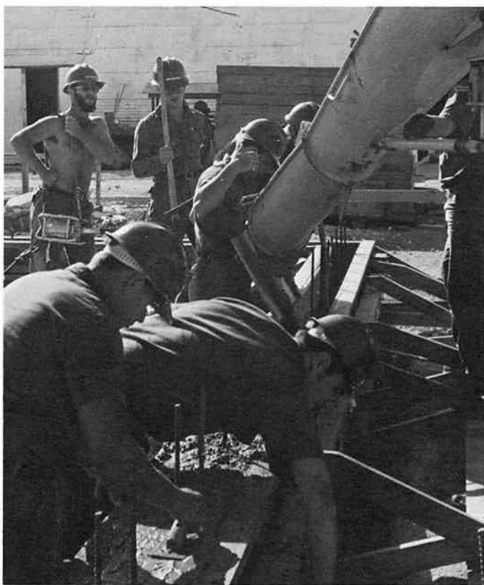
It's a thumb's up proposition for BU2 C. Aitken in placing the foundation at the new package store.
