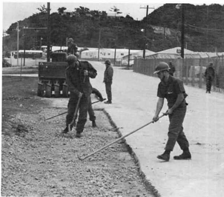
EOCN M. Kowalski (FRONT LEFT) and EOCA D. Merkle (FRONT RIGHT) improve main road at Camp Shields.
