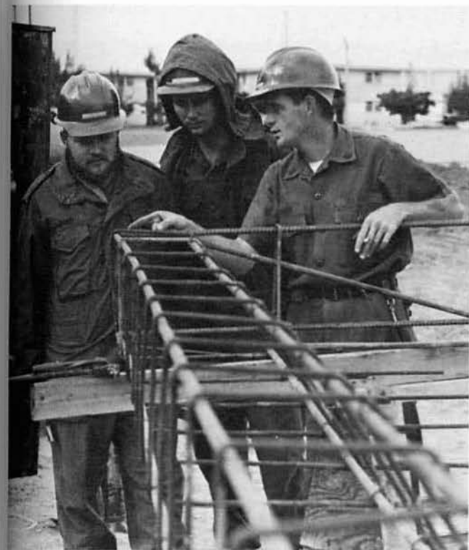
SWCN R. Flournoy (l) SWCN L. Cummings (c) and SW2 O. Barefoot combine efforts on the Package Store's rebar.
