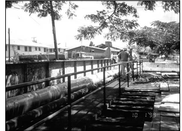
Below: The dilapidated Waipahu Depot bridge at Kapakahi Stream will be replaced by a new bikeway bridge. The State is planning a nature education facility for children at Pouhala Marsh.
