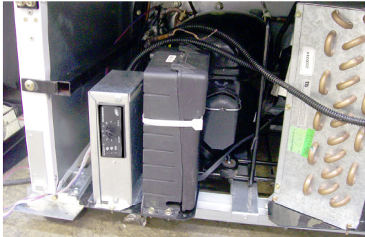
Safe-NET III Controller Location
