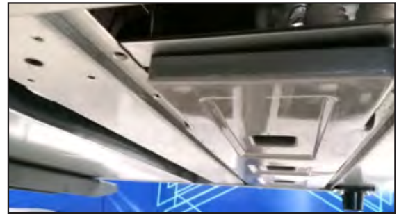
Condensate Pan Installed
