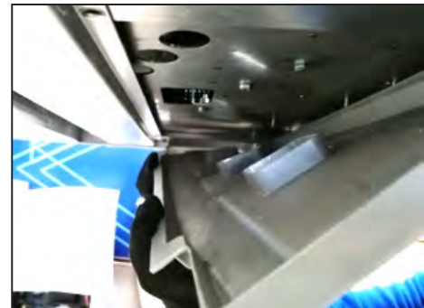
Condensate Pan Removed
