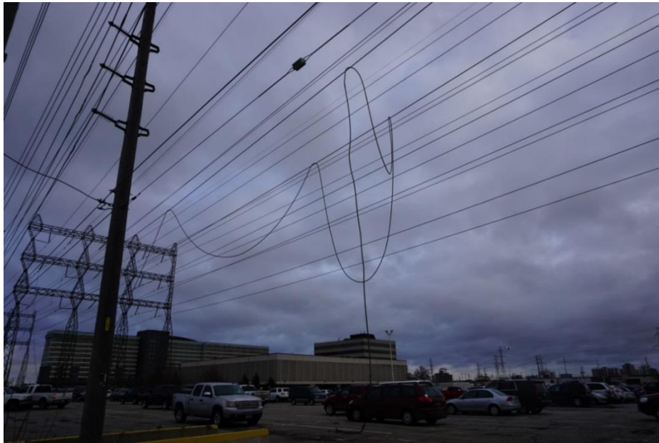
10 Figure 4: V76R Insulator Failure
