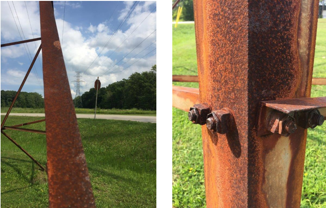
4 Figure 1: Steel Structures in the Sarnia area exhibiting heavy pitting corrosion
