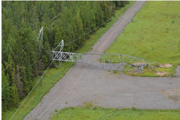
7 Figure 1: 2016 L20D (Kipling GS x Harmon Jct) Steel Structure Failure Due to Windstorm
