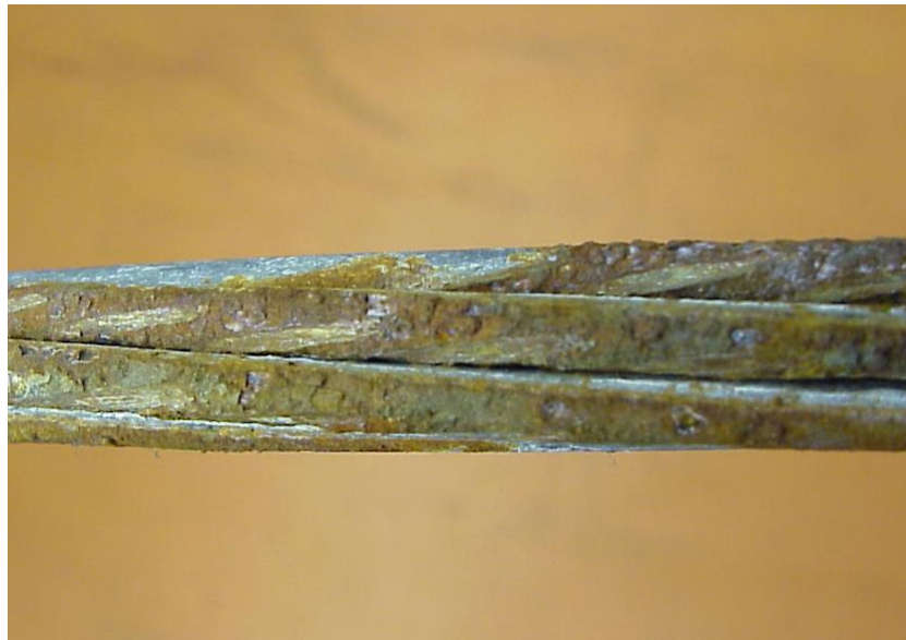
7 Figure 1: Dissected ACSR Conductor from Circuit B5C Revealing Deteriorated Core Strands with 8 Pitting Corrosion
