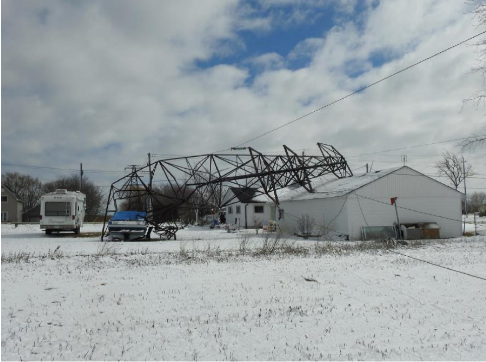
4 Figure 4: 2018 K2Z (Haycroft DS x Belle River Jct) Steel Structure Failure
