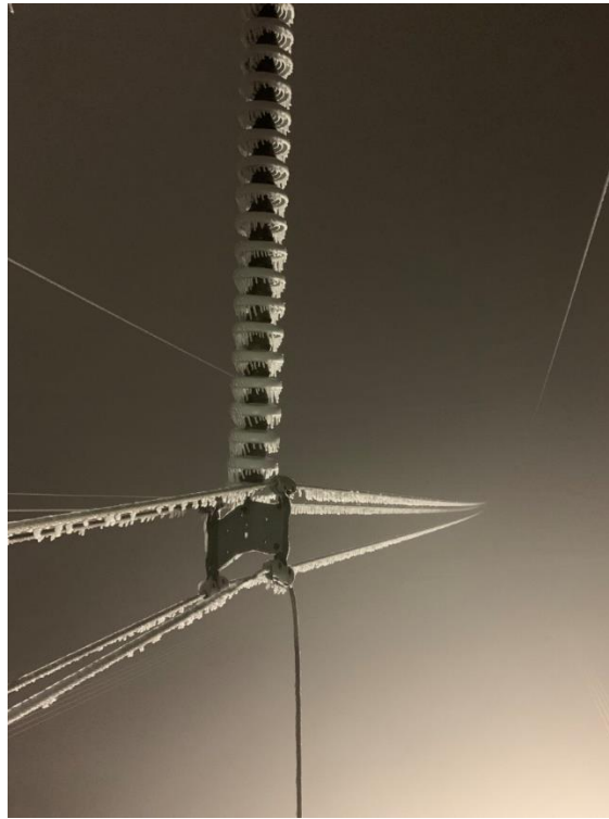
Figure 15: Broken conductor on ice accumulated 500 kV circuit B501M
