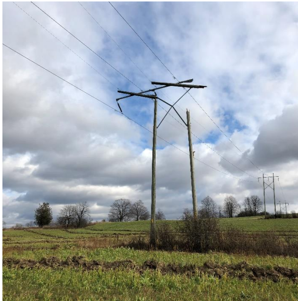
Figure 24: Failed Wood Pole on Circuit P4S
