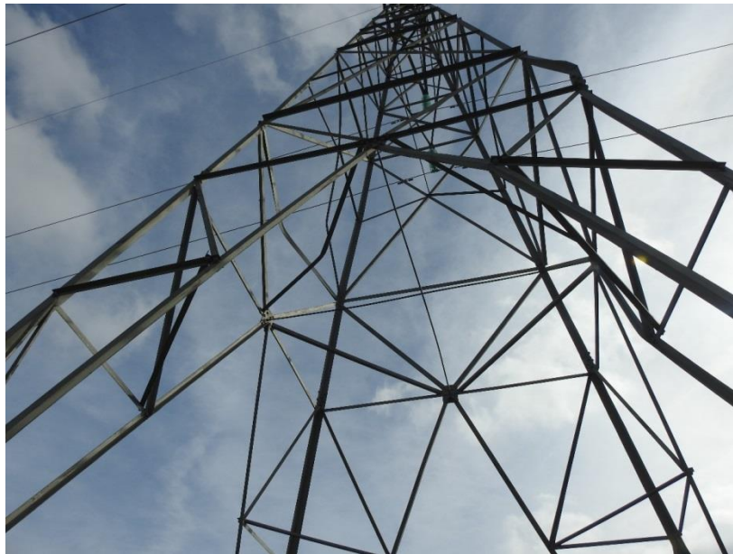
Figure 5: Bent Tower Leg (D8S Tower # 347)
