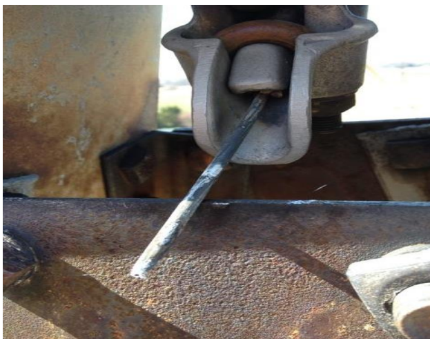
Figure 3: 2016 Shieldwire Failure on K22
