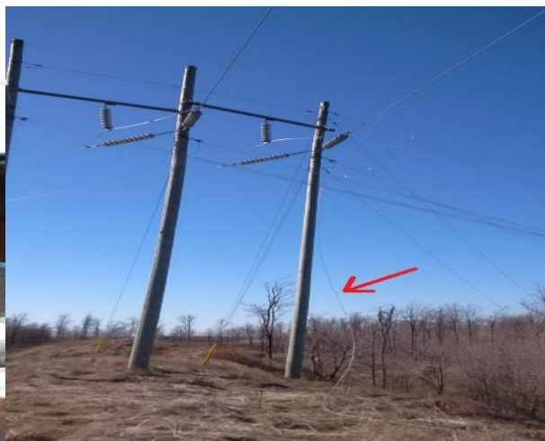
Figure 4: 2016 Shieldwire Failure on D10H
