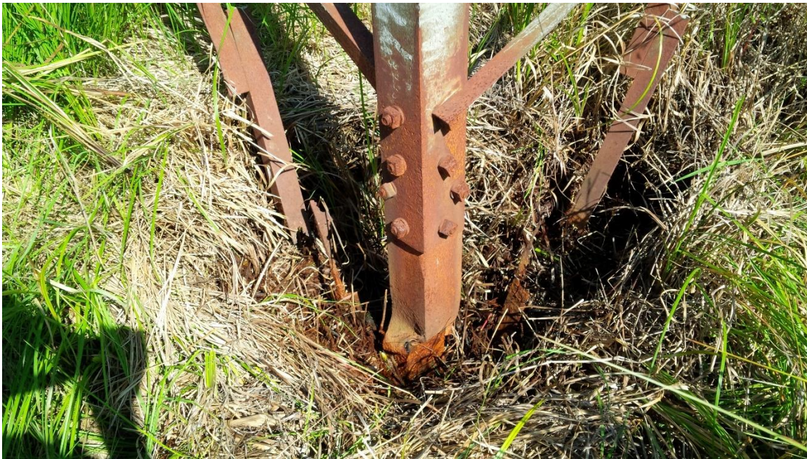
Figure 3: Leg and Diagonals are Corroded Through, Necessitating Costly Repairs (circuit D2L)
