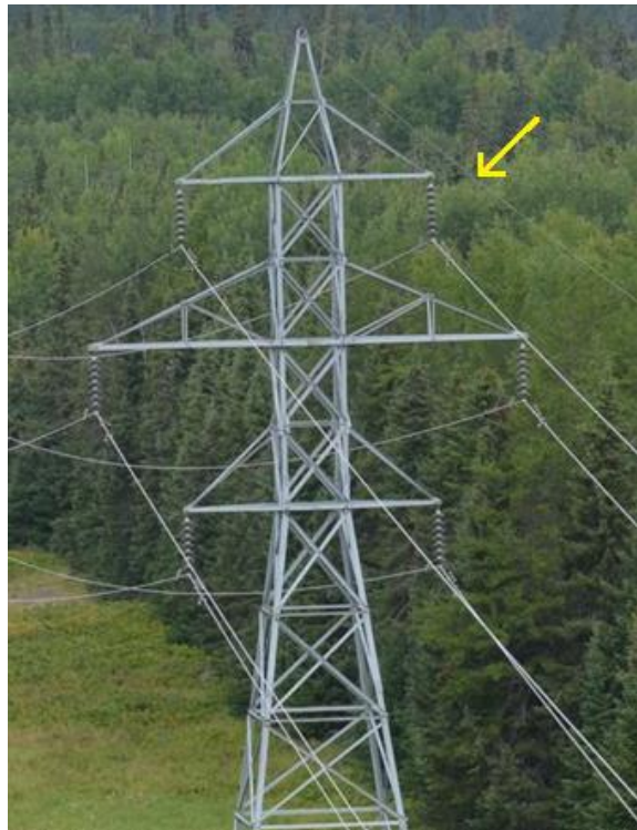
Figure 1: Transmission Line Shieldwire
