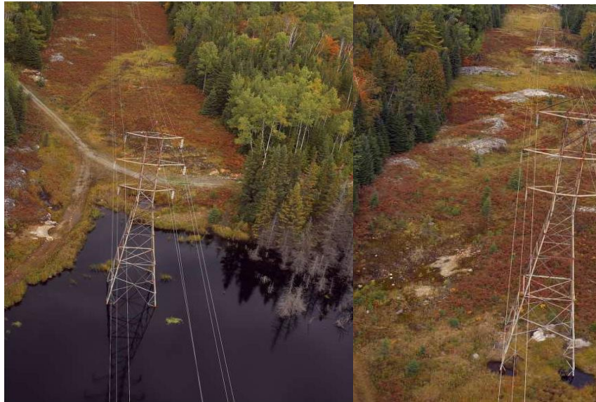
Figure 1: Towers Sitting in Water Causes the Foundations to Corrode, Leading to Towers Leaning (Circuit D2L, Near North Bay, ON)
