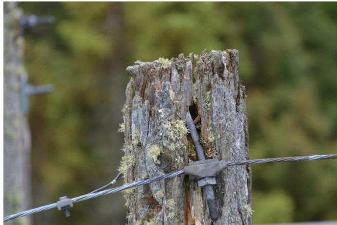
Figure 5: Rotten Pole Tops on M1T that Could Fail Imminently
