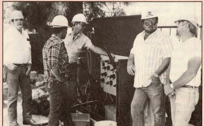
Safety Committee with D & B Electric in San Diego on an underground switch, from left: Lee Thomas, Rojo Gaerlan, Jackie Bendo, William Catalfio and P.R. James.
