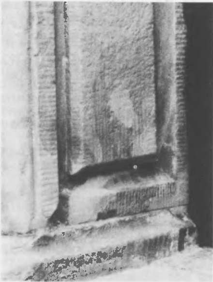
Fig.1: Dark spots still visible two years after preconsolidation treatment
