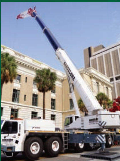
The ATF 400G-6 was rigged with 132 feet of main boom and a 76.9-foot luffing jib at a 40-degree offset.
