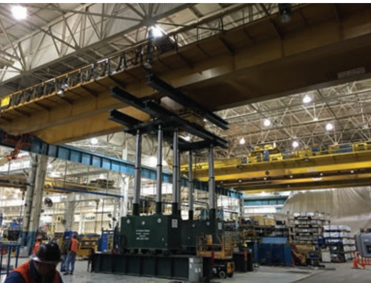
To relocate two overhead bridge cranes, International Industrial Contracting utilized two Riggers 600 EZ Lift gantry legs with a pair of headers above and below Lift System's 550-ton capacity rotation station.
