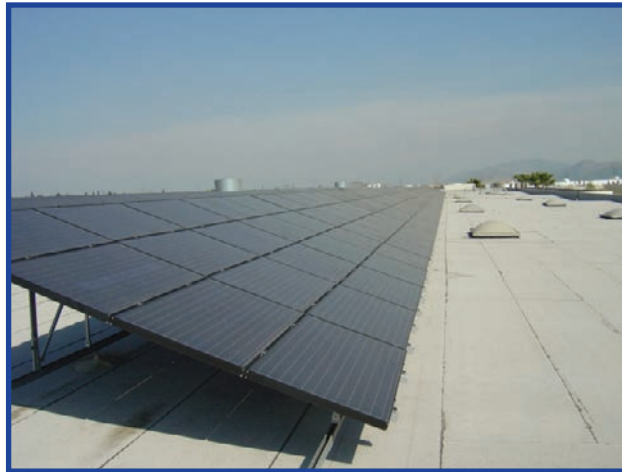
A 250 kilowatt solar photovoltaic system on the roof of a Majestic warehouse in Ontario, CA. This system eliminates 25% of the occupant's electricity bill.
