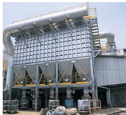
Dust collector in casting process
