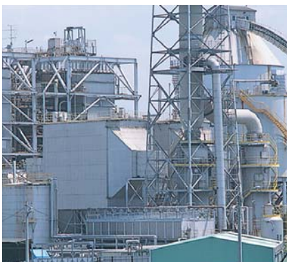
Wet-type desulfurization equipment
