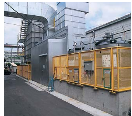
Chemical wash deodorization equipment
