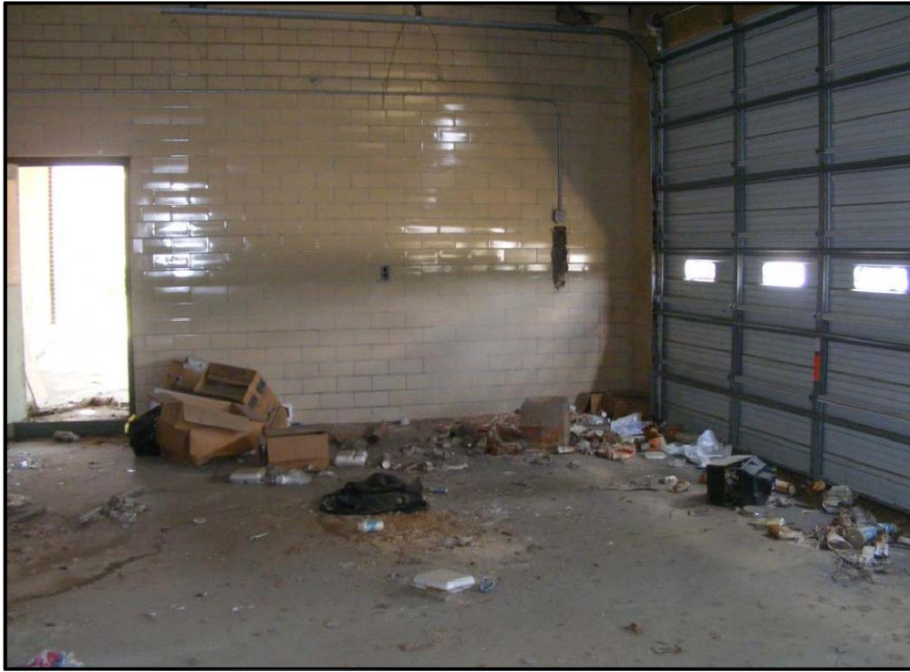
View of the interior of the former City of Jackson Fire Station #10.
