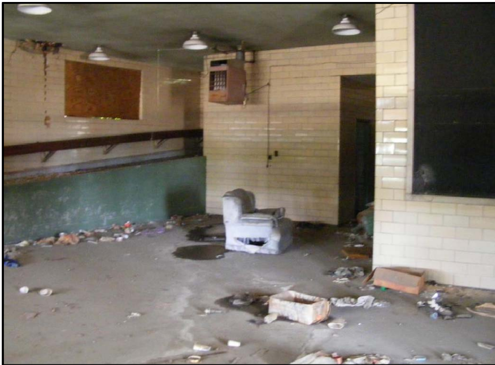
View of the interior of the former City of Jackson Fire Station #10.
