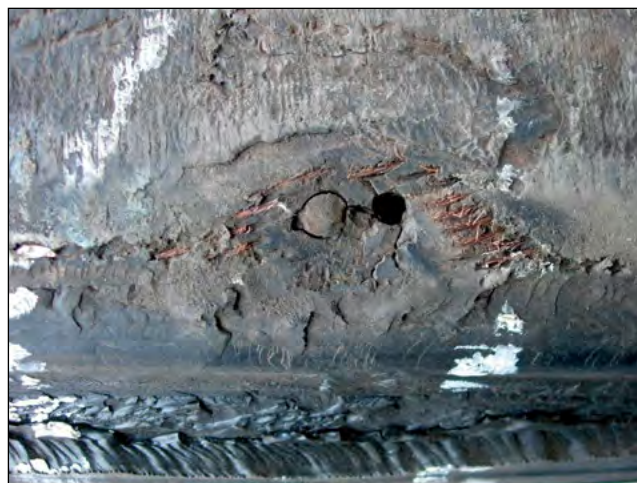
EFFECT: Missed Nail Hole CAUSE: Repaired from the Outside Resulting in Missed Damage
