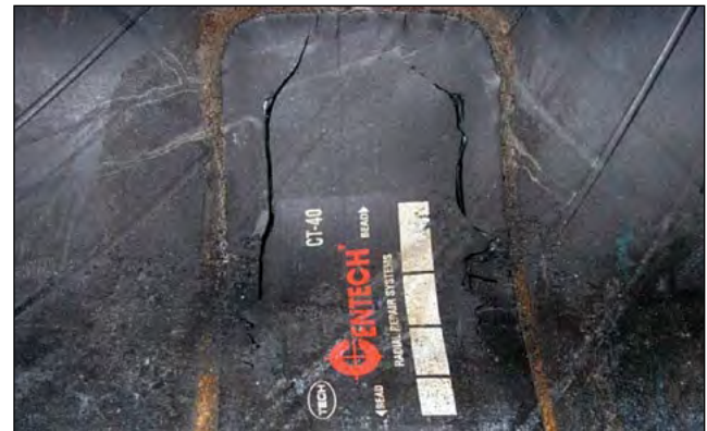
EFFECT: Crack in the Repair Unit CAUSE: Improper Repair or Improper Repair Procedures
