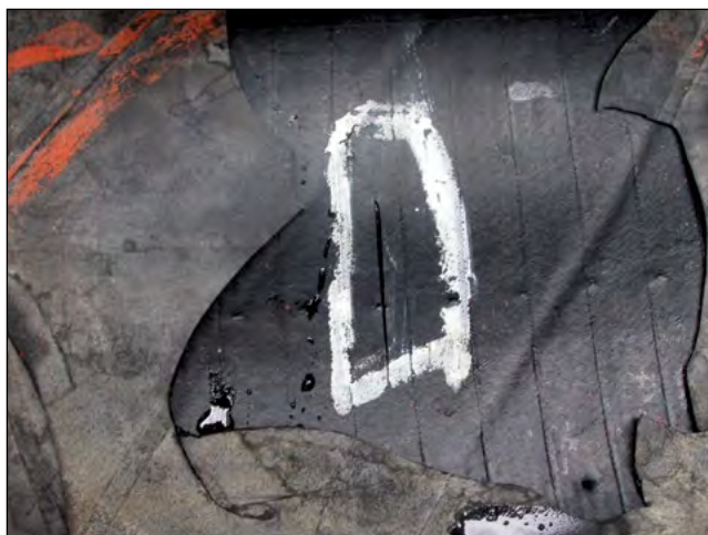
EFFECT: Radial Liner Split CAUSE: Due to Impact
