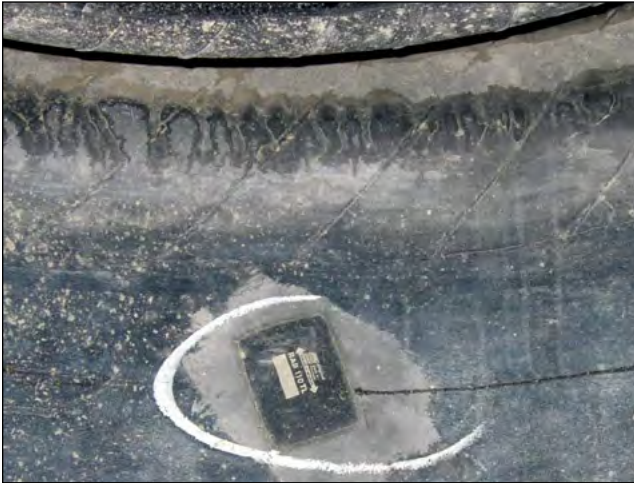
Improperly Aligned Repair (Note that the arrows on the patch do not point toward the beads.)
