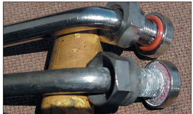
Note Corrosion On Bottom Valve
