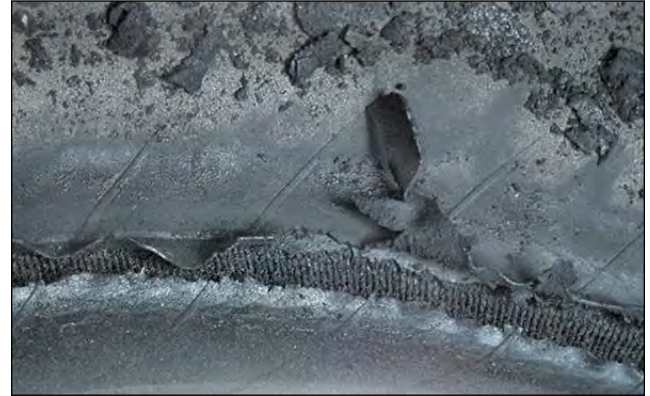
Inner Liner Damages
