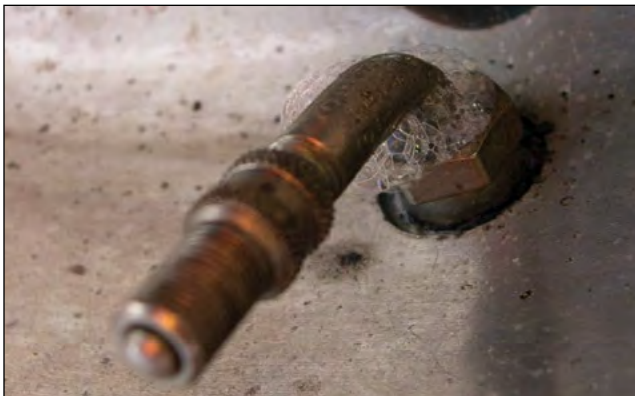
EFFECT: Leaking Valve, Grommet, or Wheel CAUSE: Improper Installation - Torque, Lubrication, Corrosion
