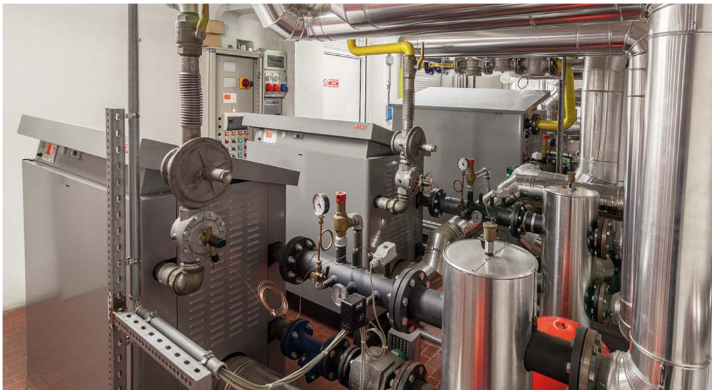
INSTALLATION IN BOILER HOUSE • ITALY
