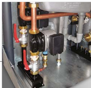
Pumps and gate valves
