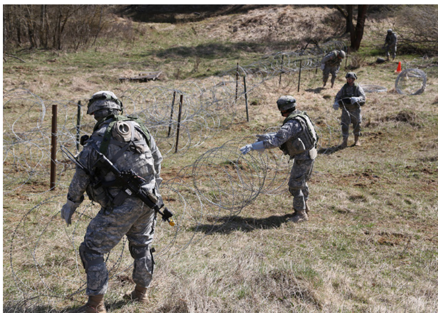
Figure 2. Soldiers from Regimental Engineer Squadron, 2 nd Cavalry Regiment, set up a concertina-wire obstacle while constructing defensive obstacles during Exercise Saber Junction 2015 at JMRC in Hohenfels, Germany. Saber Junction prepares NATO and partner-nation forces for offensive, defensive and stability operations and promotes interoperability among participants. Saber Junction 2015 had more than 4,700 participants from 17 countries. (Photo by SPC Tyler Kingsbury)
