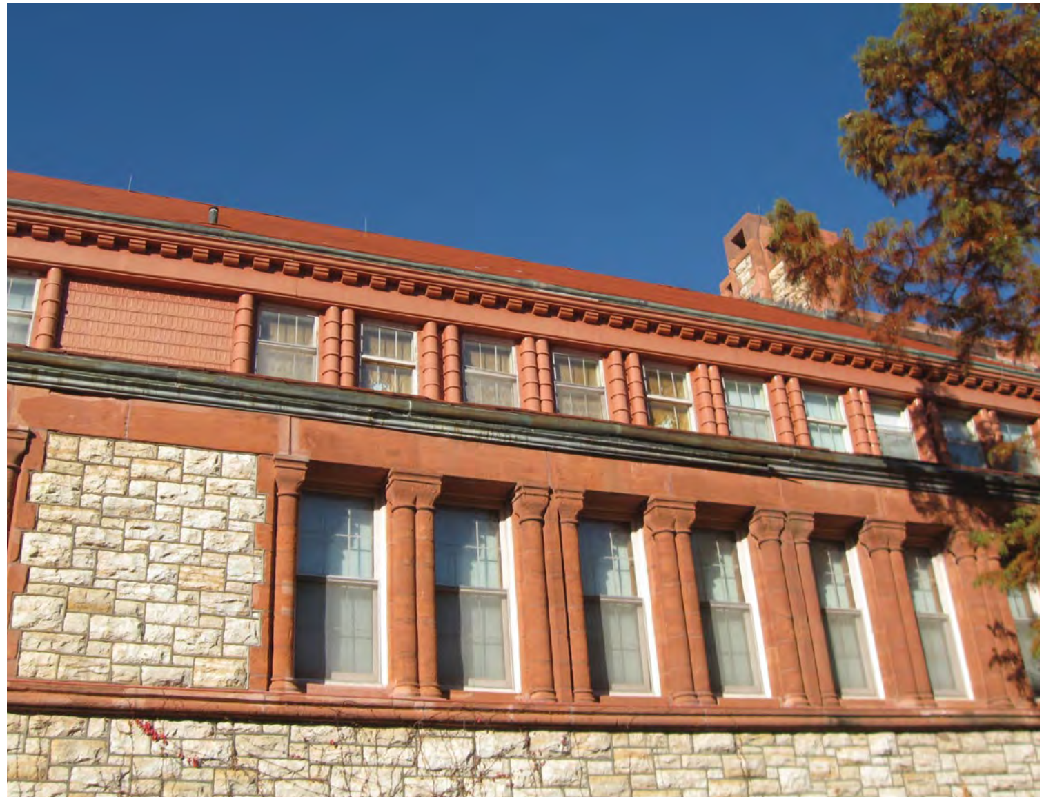
[6] Preliminary work before starting restoration revealed that the columns and the decorative shingles ornamenting the top floor of this historic building were fabricated of metal to imitate the red sandstone used elsewhere on the building.
