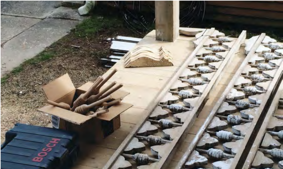
[5] New wood trim pieces were milled to match the few remaining historic features to replace those that were missing.
