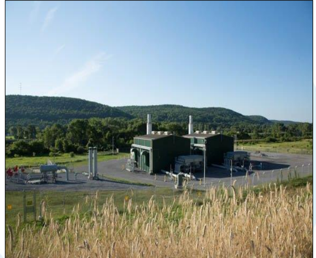
Hinsdale Compressor Station, Hinsdale, NY (Cattaraugus County)
