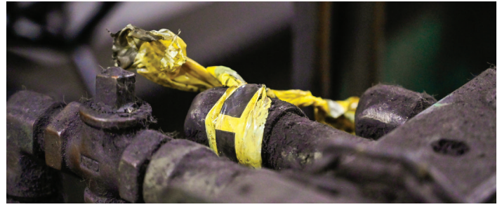
Marker identifying air leaks at the Republic Steel facility. Each repaired leak will save the company approximately $1,500 a year.
