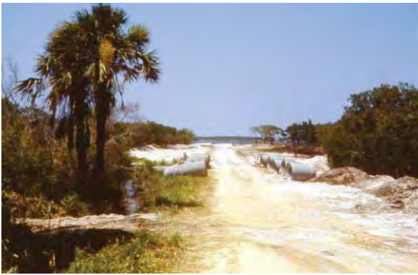
FIGURE 2-41. View north into parking area at start of construction, 1950; concrete pipe is for building culverts beneath the road. (DESO Archives)
