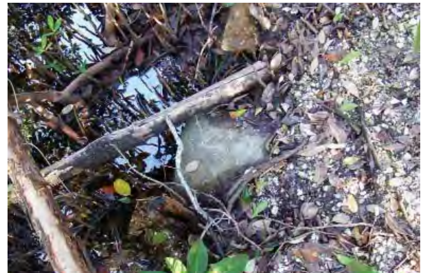
FIGURE 3-176. Detail of pipe culvert under shell path, channel crossing under south loop trail.
