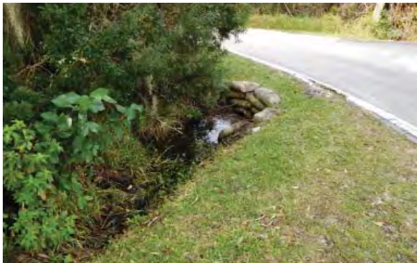
FIGURE 3-172. Channel along west edge of entrance road, culvert under maintenance drive, view west.
