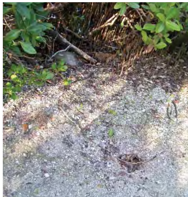
FIGURE 3-74. Path subsidence, south loop trail at culvert.
