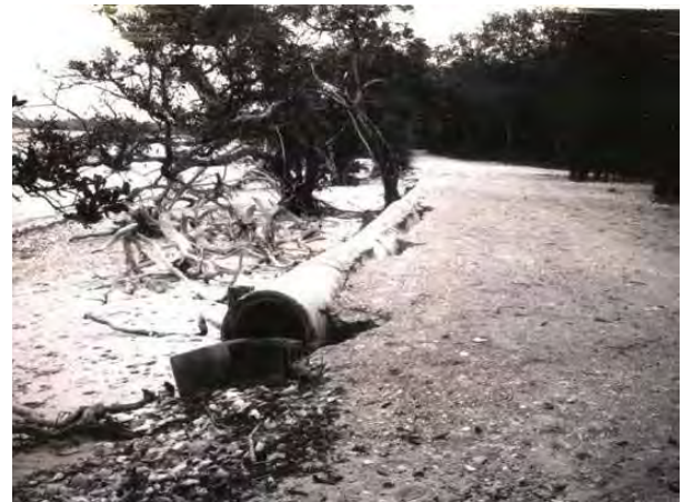
FIGURE 2-77. Culvert bulkheading, photographed after storm damage, November 1968. (DESO Archives)
