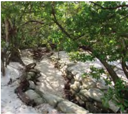
FIGURE 3-177. Channel on north shore, approximately 50 yards east of visitor center, view southeast.
