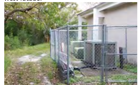
FIGURE 3-108. Equipment enclosure east of building, view south.
