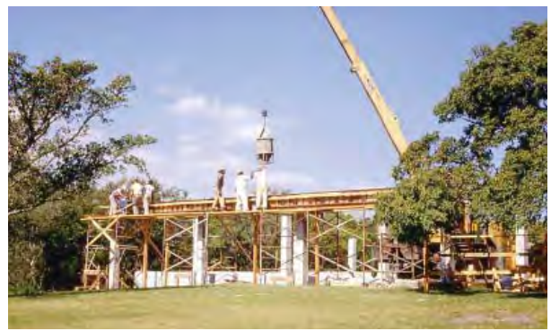
FIGURE 2-91. Visitor center construction, 1967-1968; forming and pouring concrete columns and beams. (DESO Archives)
