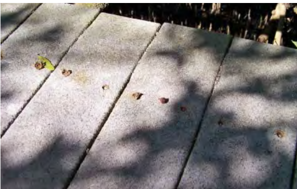
FIGURE 3-80. Failed deck screws.
