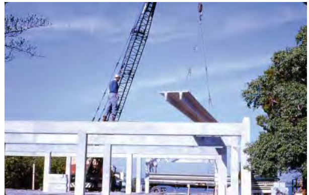
FIGURE 2-93. Visitor center construction, 1967-1968; placement of prestressed double-tees to form the building's roof. (DESO Archives)
