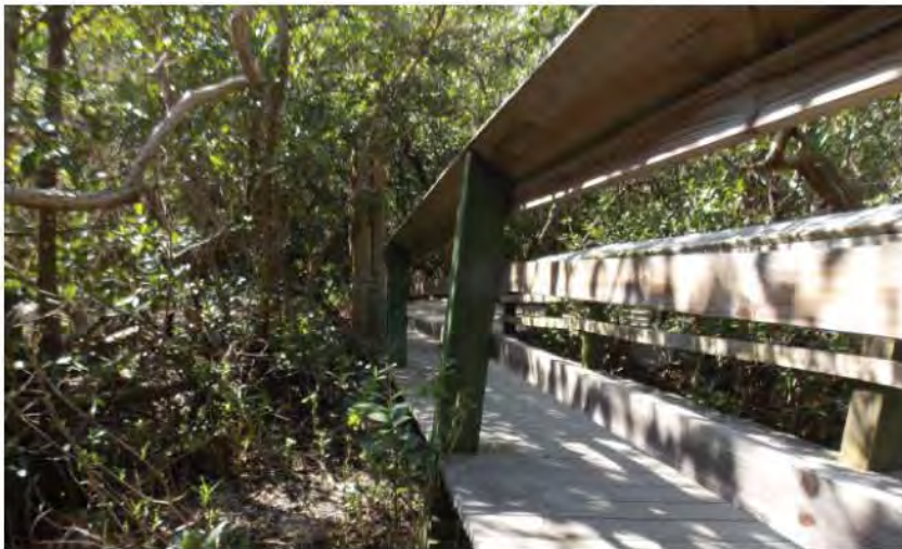
Photo 4; View of out of plumb 6x6 wood post.
