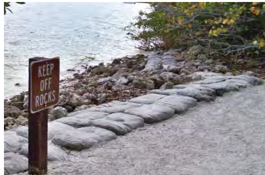
FIGURE 3-180. Rip rap and cement-bag revetment, cove trail just south of Point, view south.
