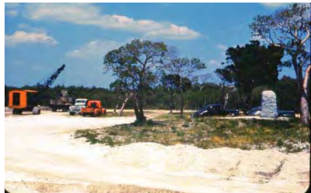
FIGURE 2-48. Fill being placed in "plaza" and beach area north of the monument, 1950. (DESO Archives)
