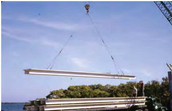
FIGURE 2-92. Visitor center construction, 1967-1968; placement of prestressed double-tees to form the building's roof. (DESO Archives)
