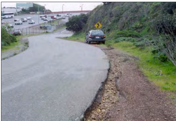
Photo 1.6. Typical unpaved shoulder parking and resultant
