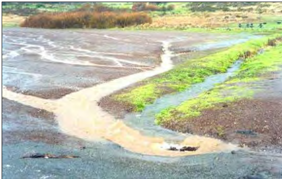
Photo 1.5. Erosion at the Rodeo Beach unpaved parking area.
