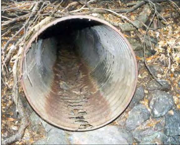
Photo 1.2. Rusted culvert under East Road.
