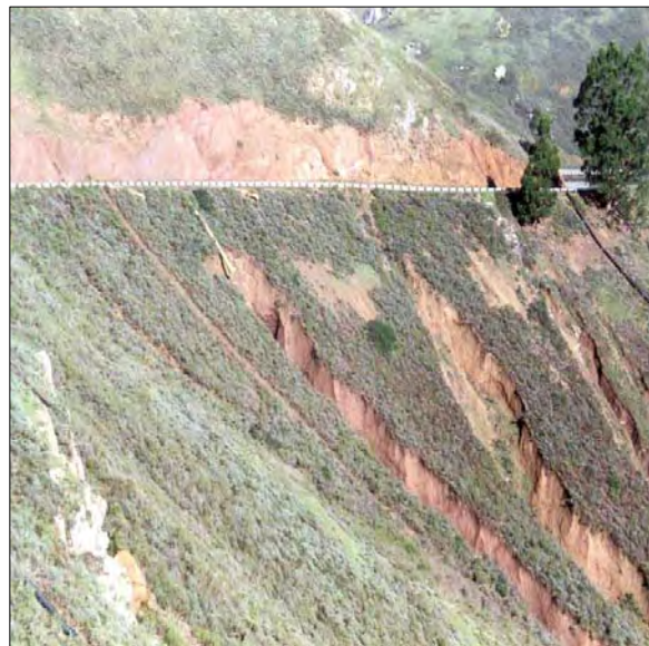
Photo 1.14 Erosion scars below Conzelman Road.
