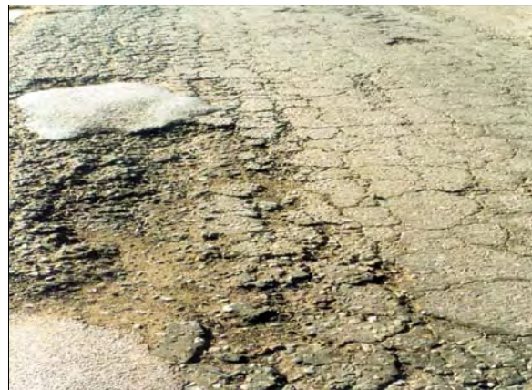
Photo 1.1. Deteriorated roadway asphalt pavement in Fort Barry.
