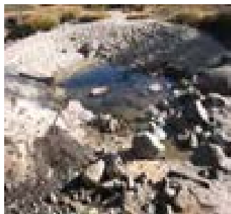
Fig. 1-18. Ponding at culvert below Budd Creek
