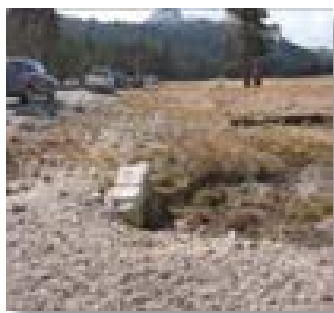
Fig. 1-17. Culvert set too low in meadow
