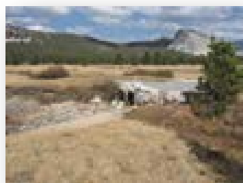
Fig. 1-26. Scour downstream of culvert on Unicorn Creek
