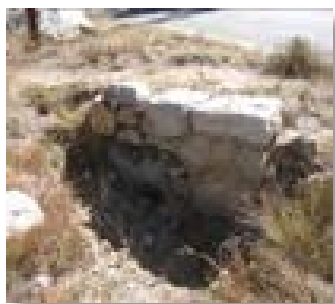
Fig. 1-16. Partially blocked culvert
